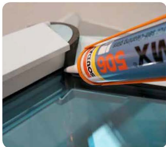
17 Seal around perimeter of the foam bung where it intersects the ridge glazing seal, glass and glazing bar top caps.
